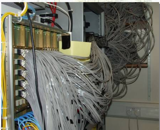
Level-1 400-Mbit/s serial 4-channel input links from programmable source modules
