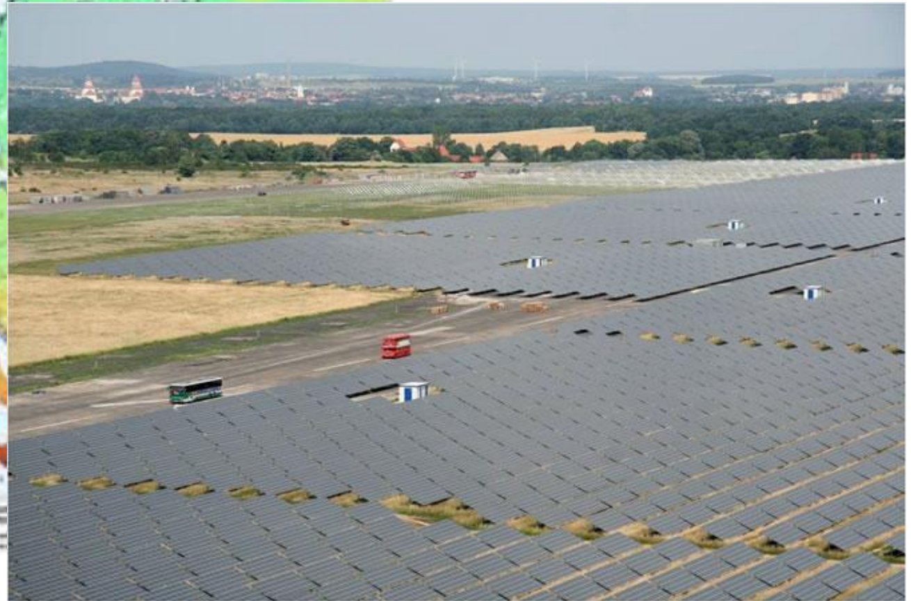
Image: Photovoltaic power station with a capacity of 40MW in eastern Germany
