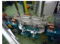
Undulator vacuum vessel installed in the ALICE beamline.
