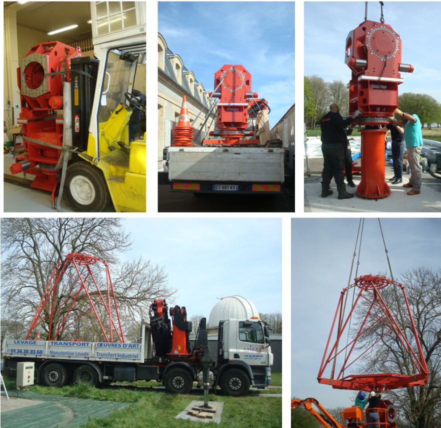
Figure 4.6 – The assembly of the telescope - From top left to bottom right: AAS removed from the integration hall by a forklift, transfer to foundation and mounted on the tower; the bottom line shows the integration of the OSS on the bosshead of the AAS.
