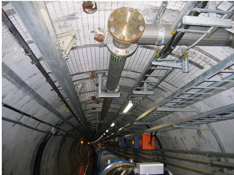
Figure 6.54: View of sector 4 showing the chain of superconducting magnets in the arc.
