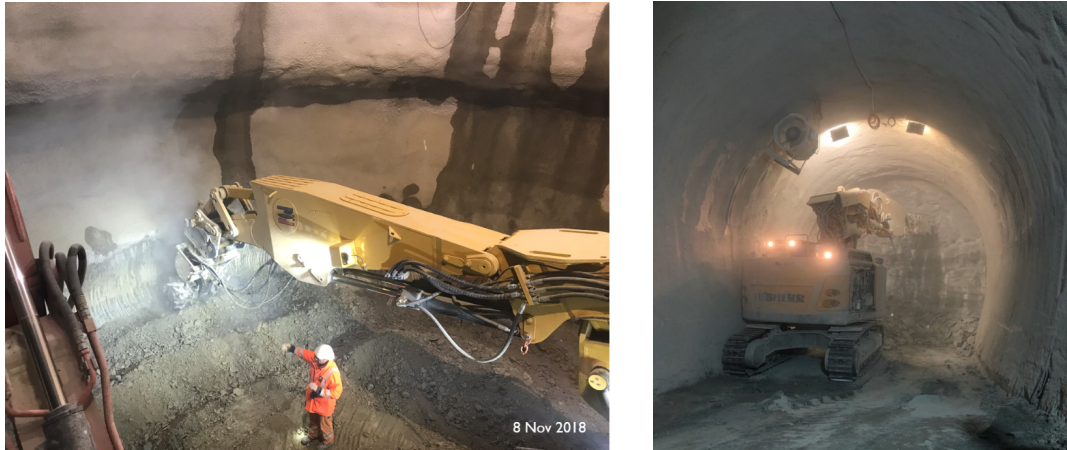
Figure 8.45: Left: Roadheader being used for shaft excavation at HL-LHC Point 1. Right: Rockbreaker used for cavern excavation at HL-LHC Point 1.
