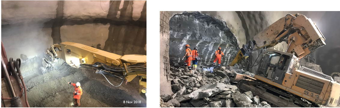
Figure 10.54: Left: Roadheader being used for shaft excavation at HL-LHC Point 1. Right: Rockbreaker used for new service tunnels excavation at HL-LHC Point 5 (Credit: Z. Arenas).
