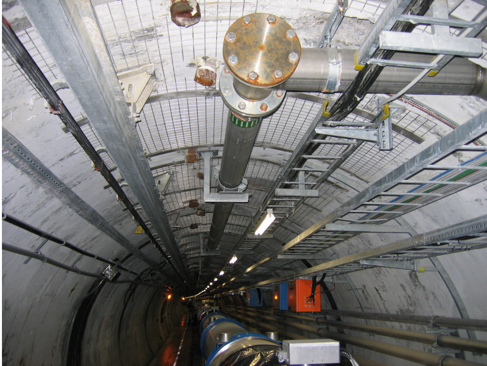
Figure 7.48: View of sector 4 showing the chain of superconducting magnets in the arc.
