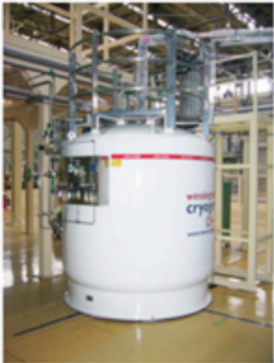
3000L liquefied helium storage vessel
