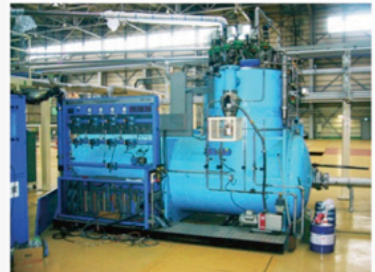
TCF200 helium liquefier/refrigerator
