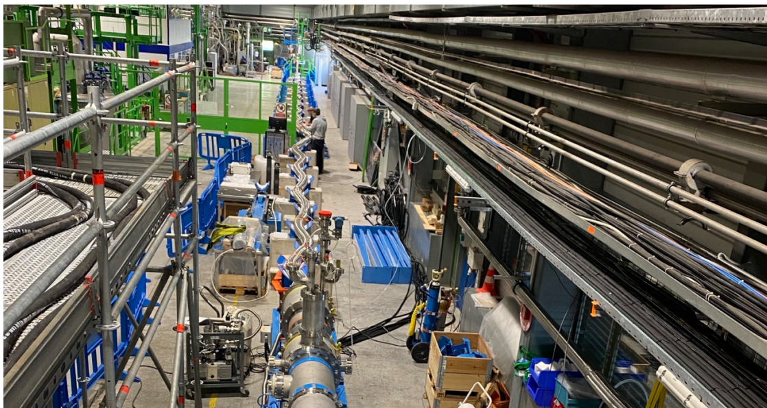
The 60-metre-long demonstrator of the superconducting electrical transmission lines for HL-LHC during testing in the SM18 hall at CERN.
