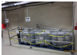
Telluric acid, underground storage
